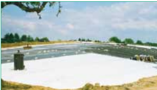
Figure 12 Composite liner with Bentofix® in a land- fill cap (landfill Bamberg, Germany).
